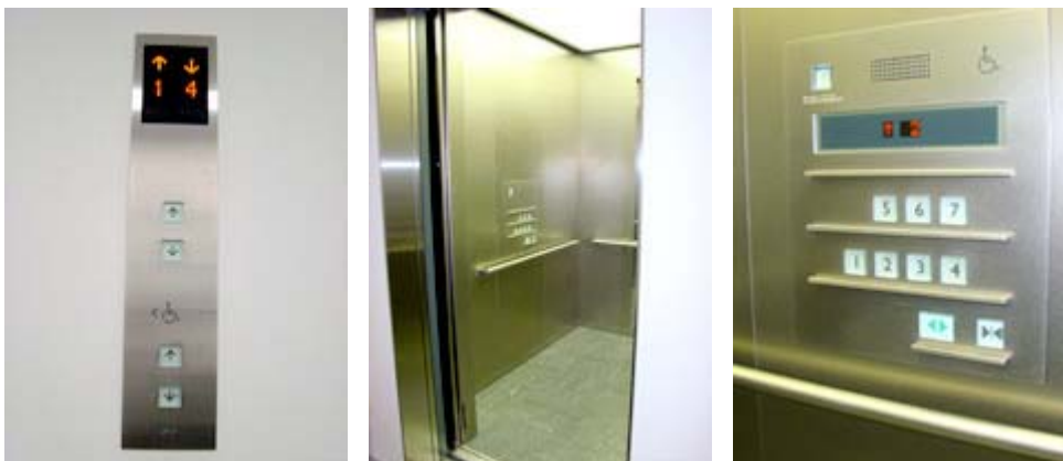
Barrier-free elevator (Advanced Technology R&D Center)
