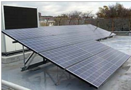
Photovoltaic panels installed on roof
